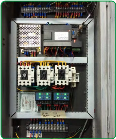
Electric Box 电箱更新
